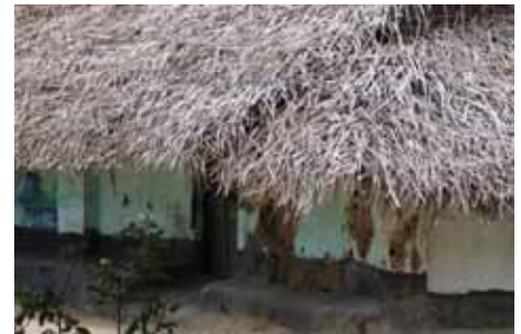
Leaky mudhuts riddled with termites.
